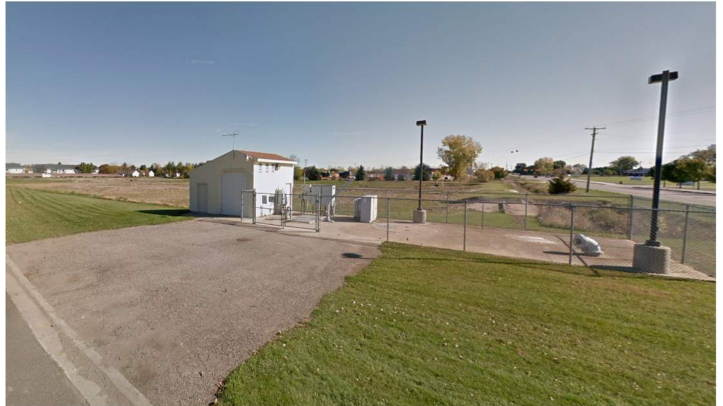
Existing Townsend Road Lift Station
