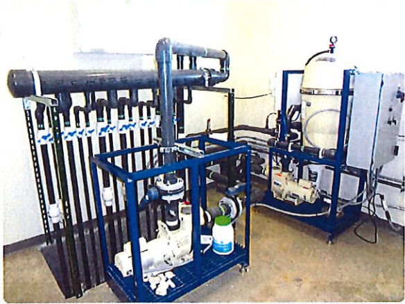
Recirculation System Equipment Room
