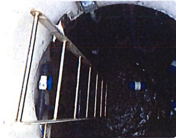
Inside of Concrete Tank with Floating Skimmer
